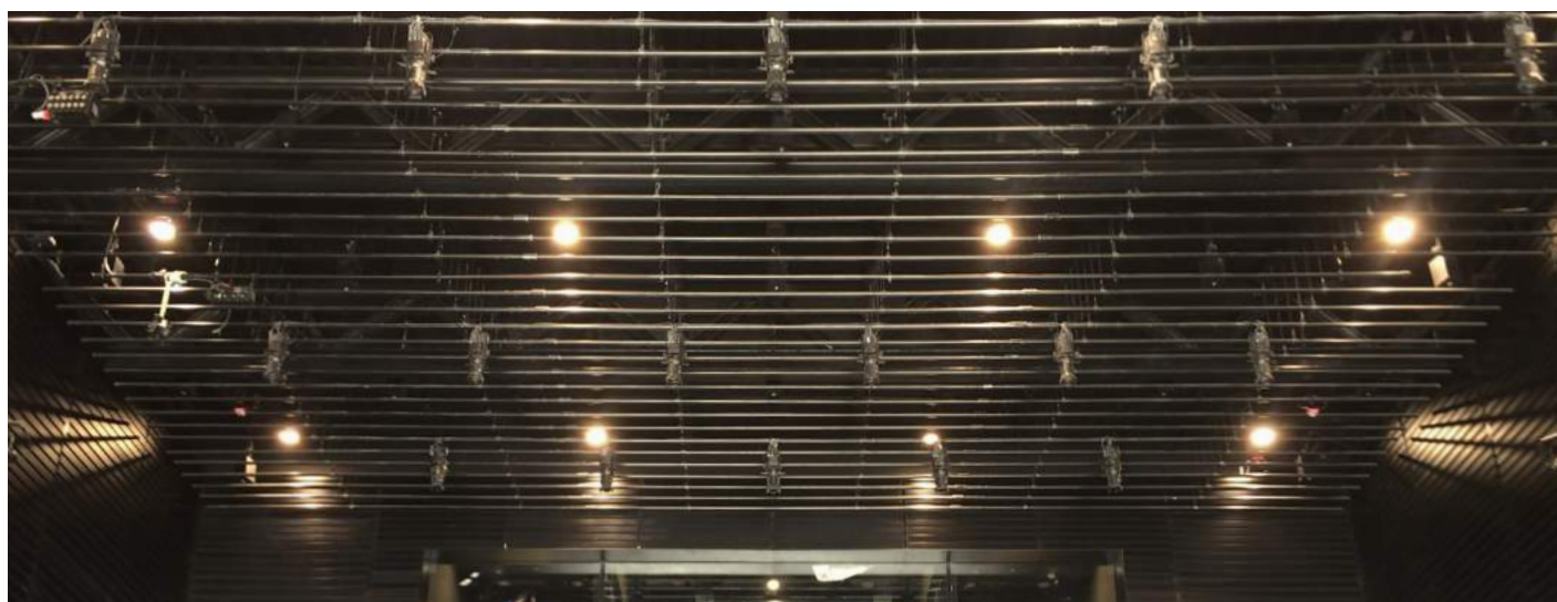
Louvre Abu Dhabi - Lineshaft System
